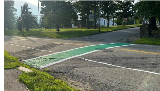
This high visibility crossing is a good approach but lacks supporting warning signage
