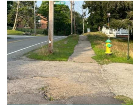
Sidewalk is in need of maintenance, very little lighting present
