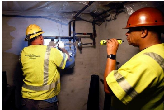
Figure 18: Render-Safe Teams Access the Interior of a Structure to Inspect the Gas Meter.
