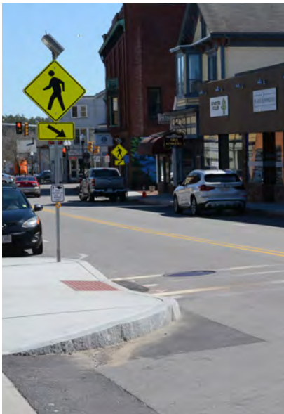
Figure 36. The new bump-outs and pedestrian crossing signs on Center Street at the approach to Thatcher's Lane make it easier for pedestrians to safely cross.
