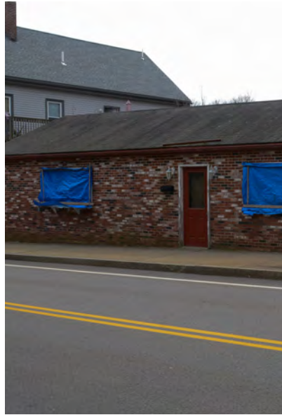
Figure D-57. The blue tarp covered windows on this Wareham Street façade contribute an unkempt look in Downtown and is calling for restoration and repair.
