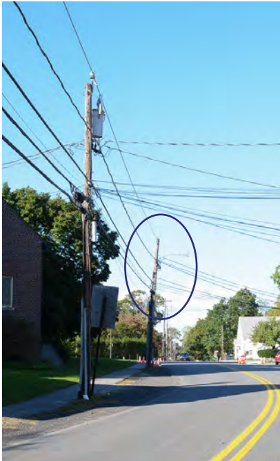
Figure 20. Streetlight on pole on Oak Street.
