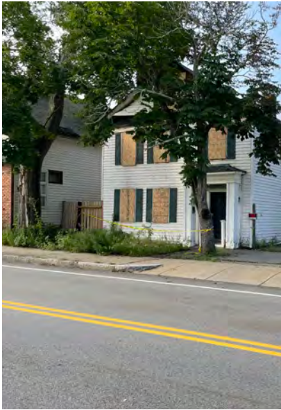
Figure D-56. A fire ravaged this building and façade. Repairs and restoration are quickly needed to avoid a blighting effect on Downtown.
