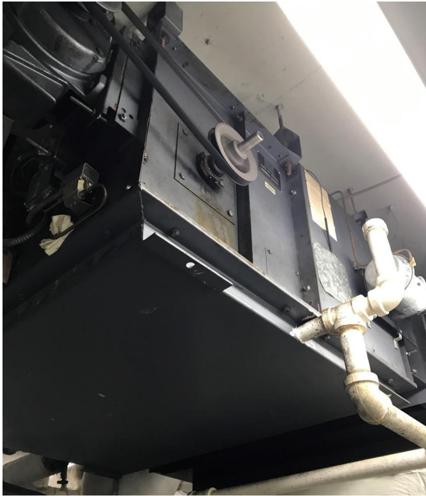
Photo 1 – Representative Air Handler
