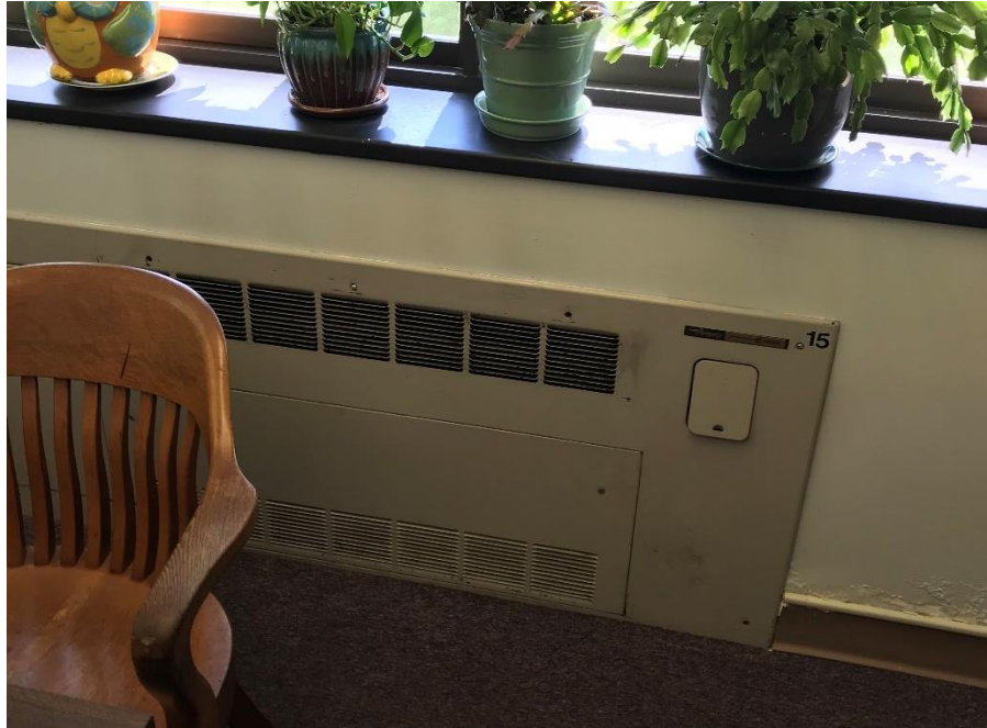
Photo 2 – Representative Fan Coil Unit
