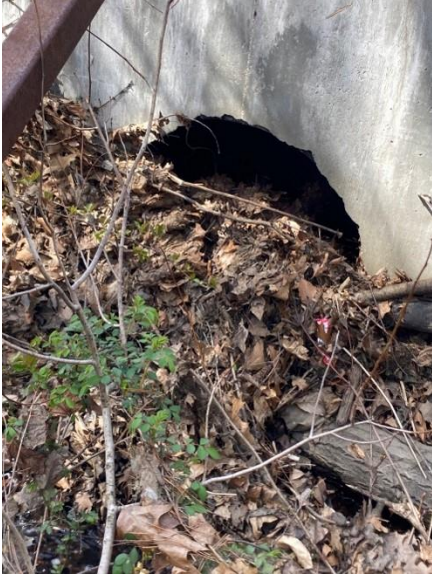
Blocked Culver, Millis, MA
