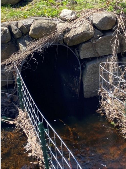
“Beaver Defender” at a Millis Culvert
