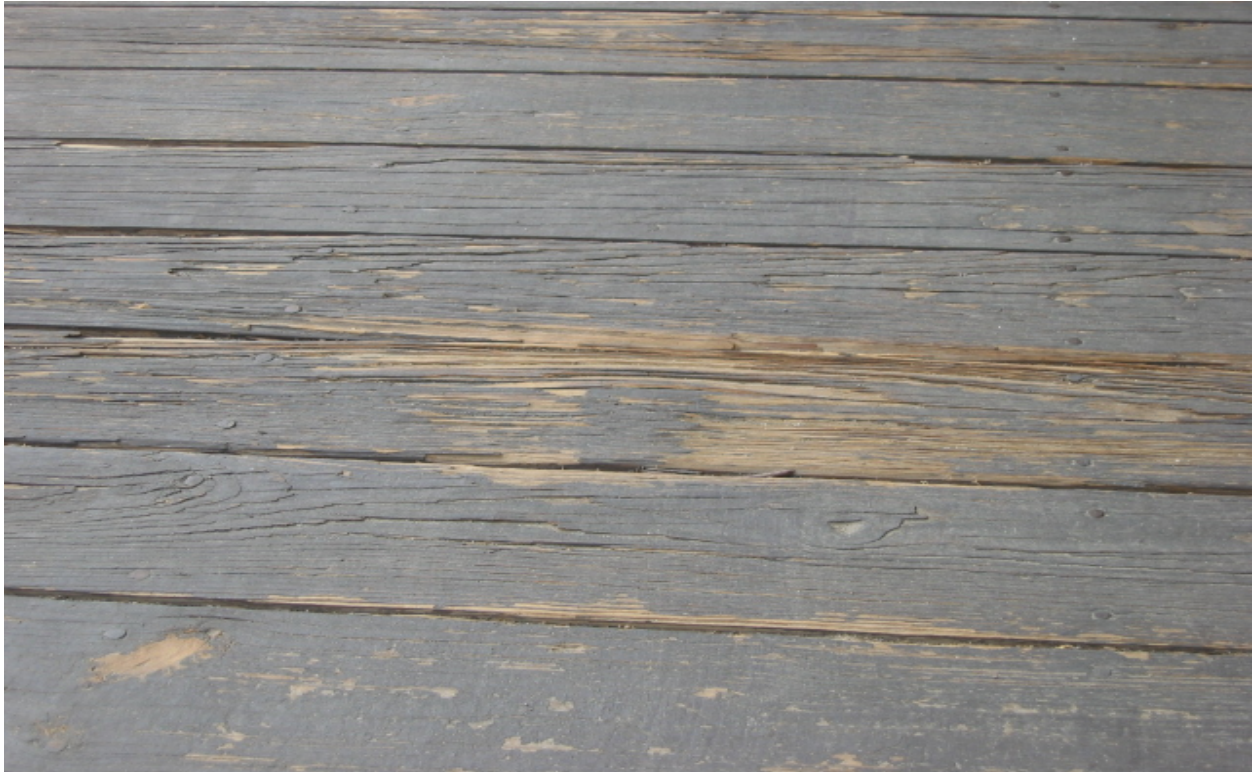
667-2 Development Canal Street # 205 Worn-Out Wooden Floor on Balcony
