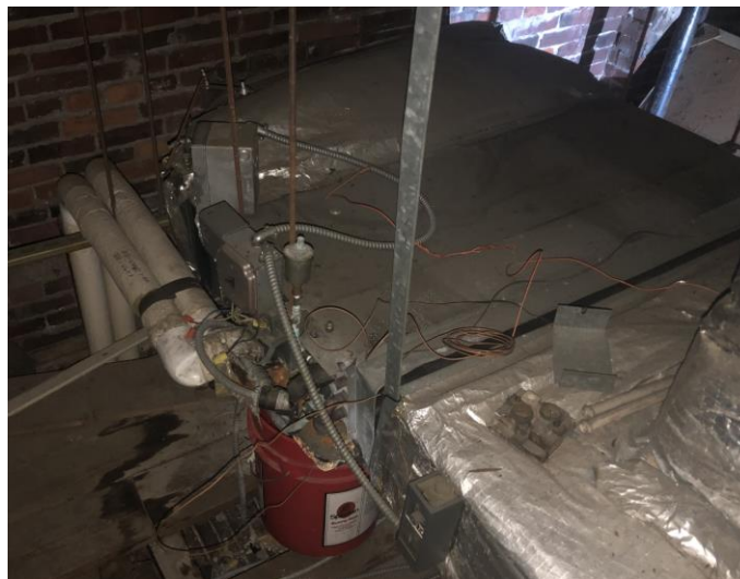
Photo 1 – Representative Makeup Air Unit
