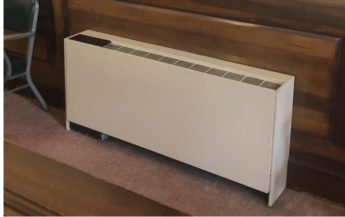
Photo 2 – Representative Fan Coil Unit
