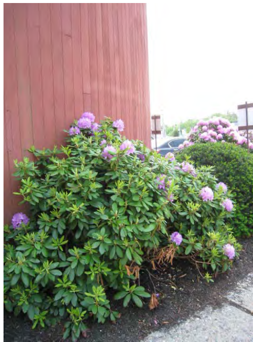
Shrubs growing close to the exterior of the building
