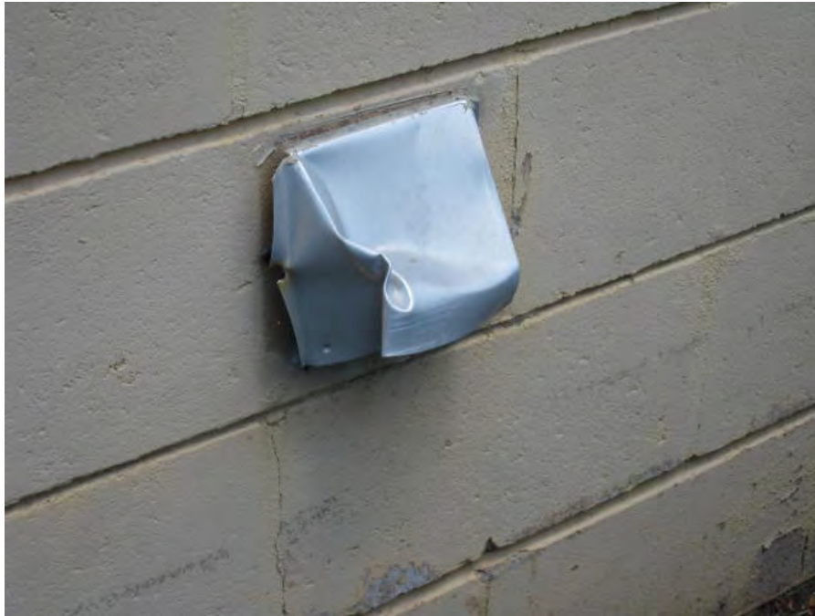
Damaged vent on exterior of building
