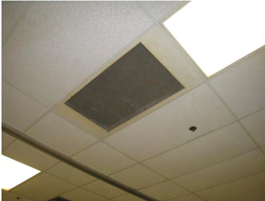
Ceiling-mounted exhaust vent
