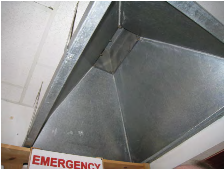
Exhaust hood structure in the cosmetology storage area
