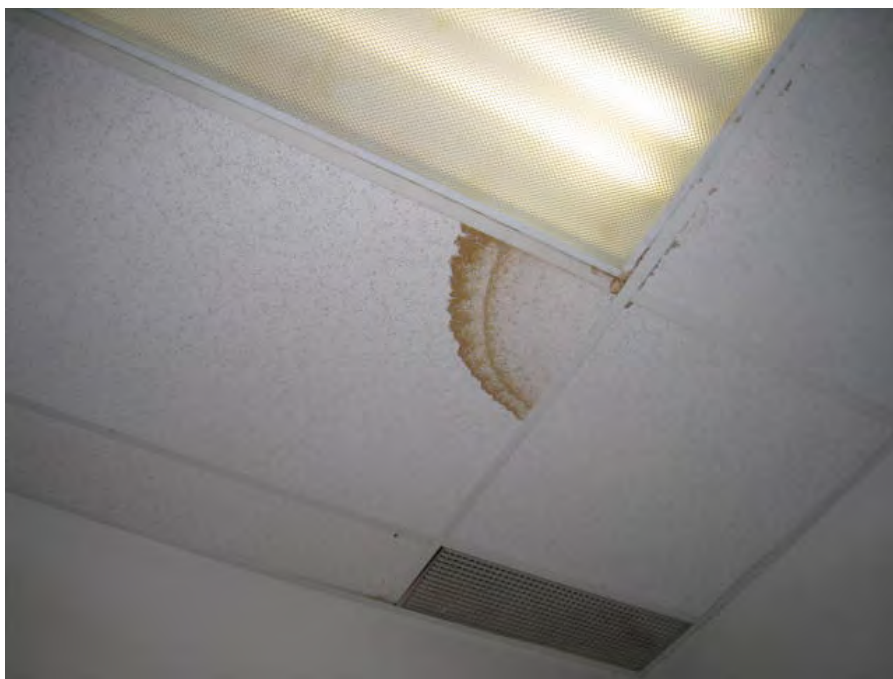
Water-stained ceiling tile
