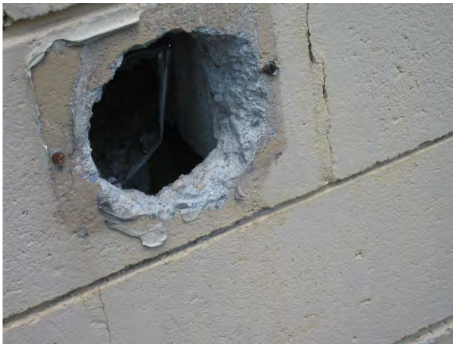
Missing vent cover/hole in exterior wall
