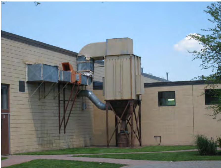
Exhaust system for carpentry area
