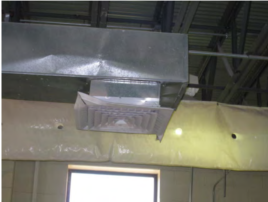
Supply vent in a workshop area
