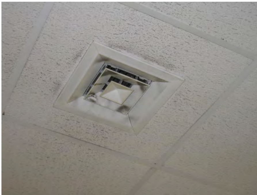
Supply vent in a classroom/office area, note dust on louvers
