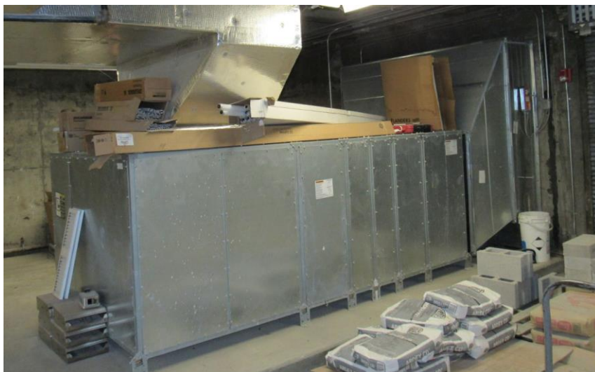
Photo 1 – AHU-1 Air Handler
