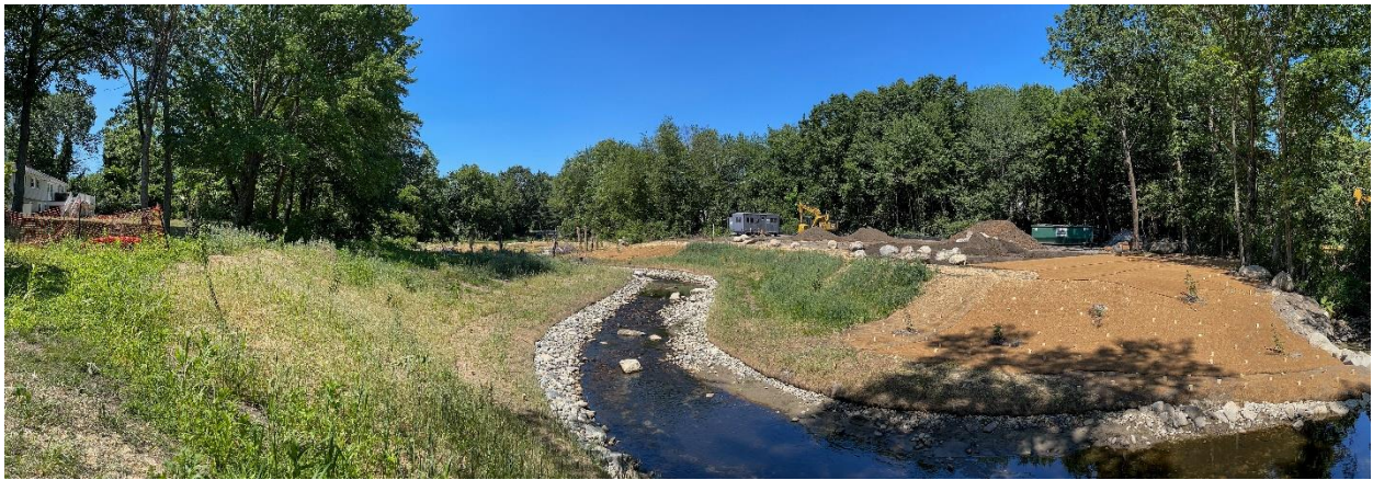
Mill Pond following dam removal and channel reconstruction. June 2022. PC: Sterling Worrell
