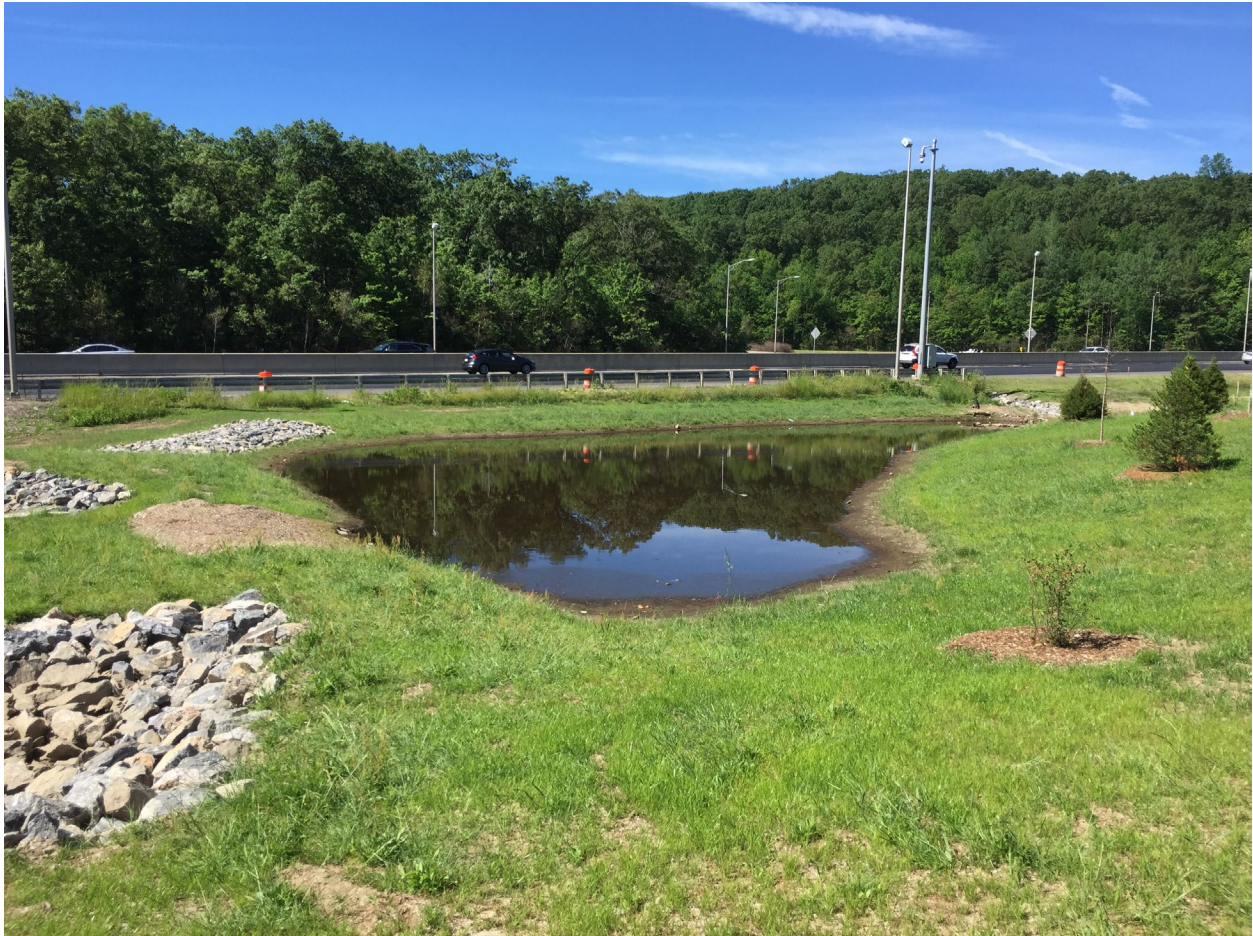
Infiltration Basin on I-90 treating stormwater discharge to Dorothy Pond in Millbury, MA.
