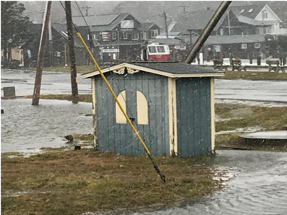
FIGURE 1 FLOODING AT LAKE AVENUE PUMP STATION (THIS IS ONE OF THE TWO PUMPSTATIONS THAT WILL BE SERVED BY THE PROPOSED ELEVATED GENERATOR).
