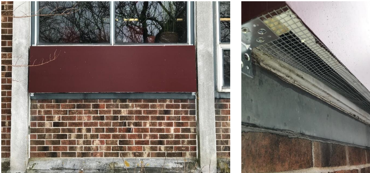
Photos 3 and 4 – Outdoor Air Intakes Boarded Over
