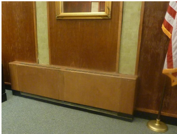
Photo 1 – Representative Unit Ventilator
