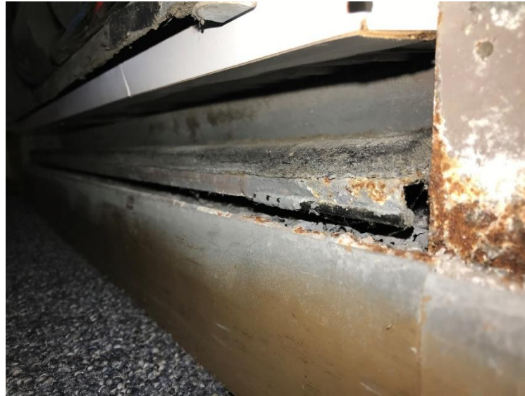
Photo 2 – Non-Functional Outdoor Air Damper
