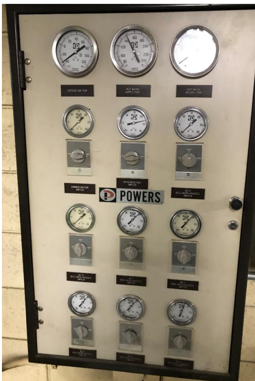
Photo 5 – Pneumatic Control Panel
