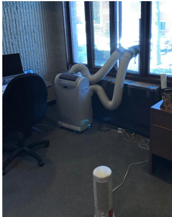
Photo 4 – Typical FCU / Portable Heat Pump
