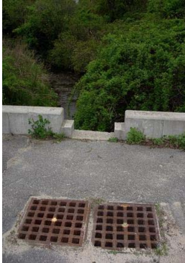
4. Unfenced 6 to 10 foot drop by culvert at Glen and Ripley Streets.
