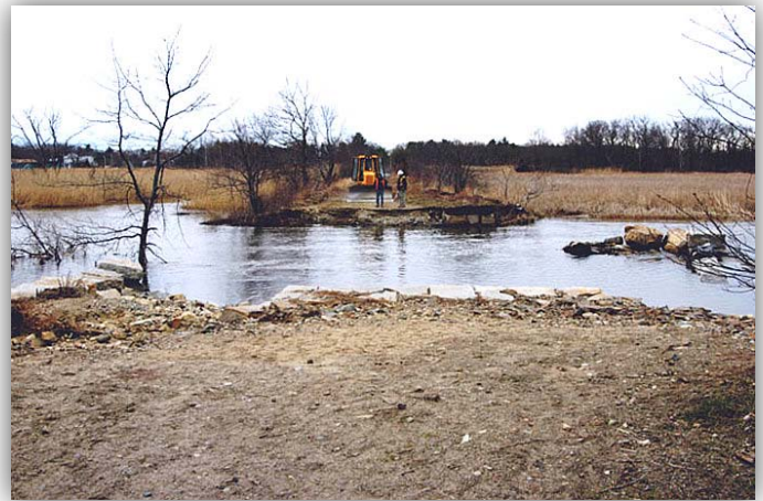
Breach in the Town Creek railroad dike following a strong spring storm in 2007.
