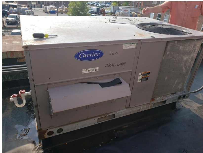
Photo 1 – Representative Rooftop Air Handler
