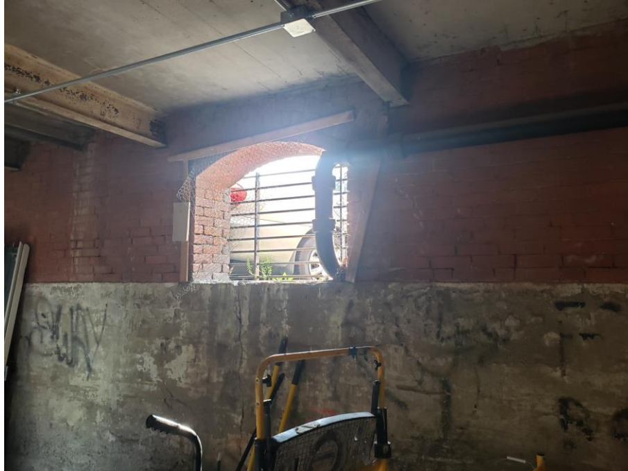
Photo 1 – Opening From RTU-7 Room to exterior. Parked Car Visible.
