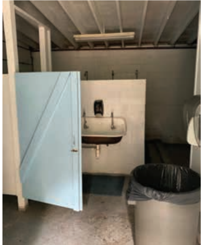
Figure 2-104. Image showing conflict between the restroom's toilet partition door swing and sinks.
