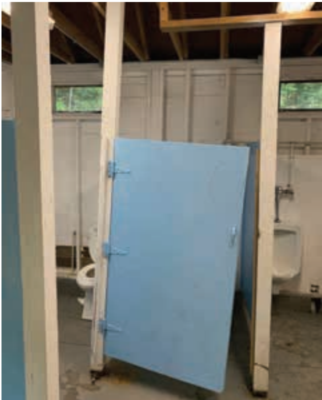
Figure 2-86. The interior conditions of the restroom facility show signs of disrepair, including failing toilet stall doors.
