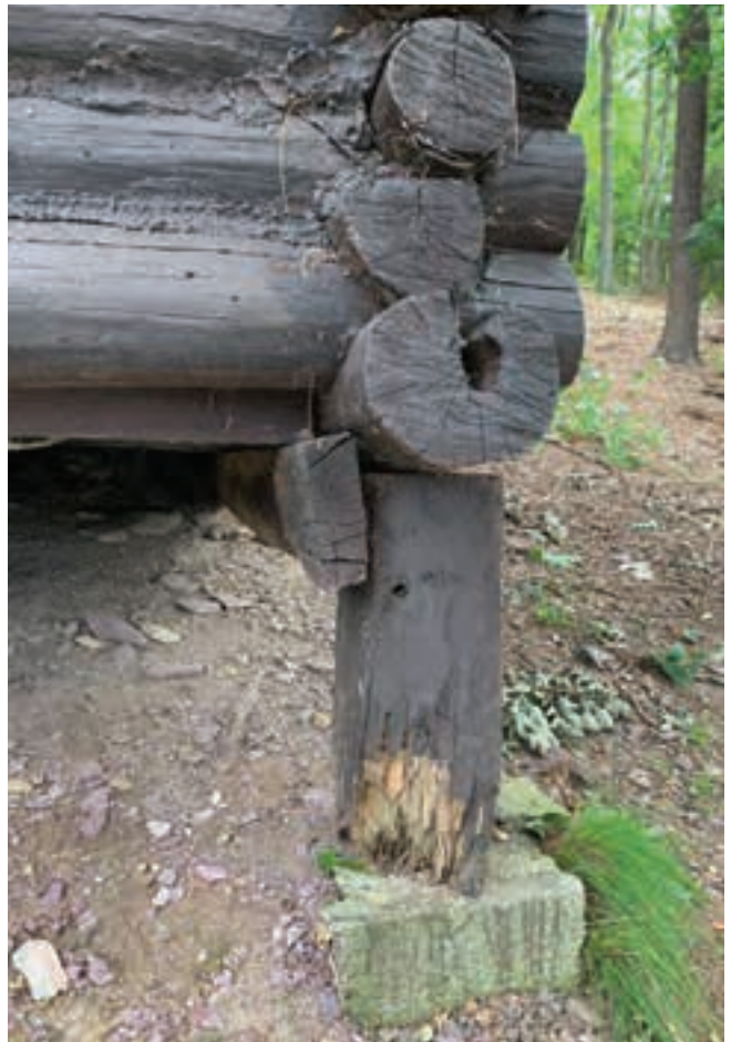
Figure 2-51. Structural degradation of Folsom cabin's support posts.
