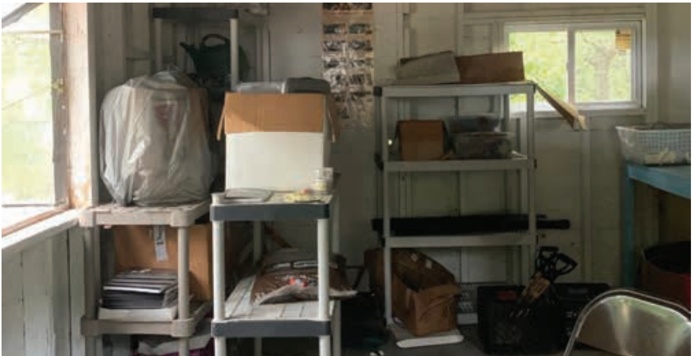
Figure 2-92. The Science Cabin's interior condition showing exposed wood stud framing and wood board sheathing
