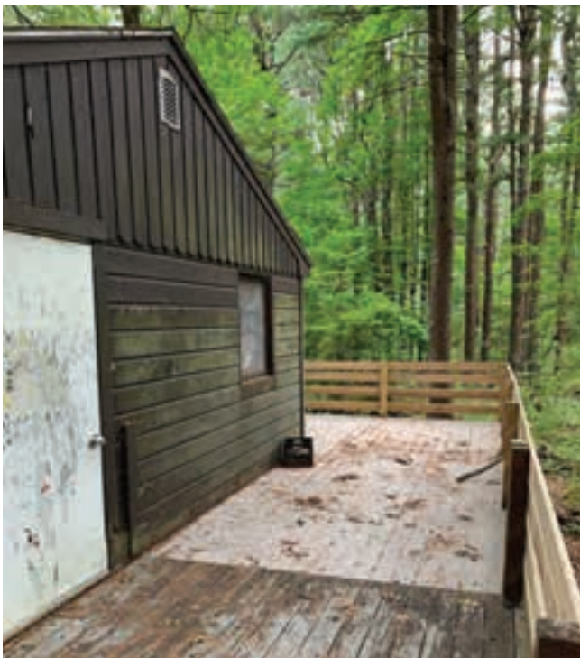
Figure 2-90. The back deck showing a more recent expansion or replacement of deteriorated materials
