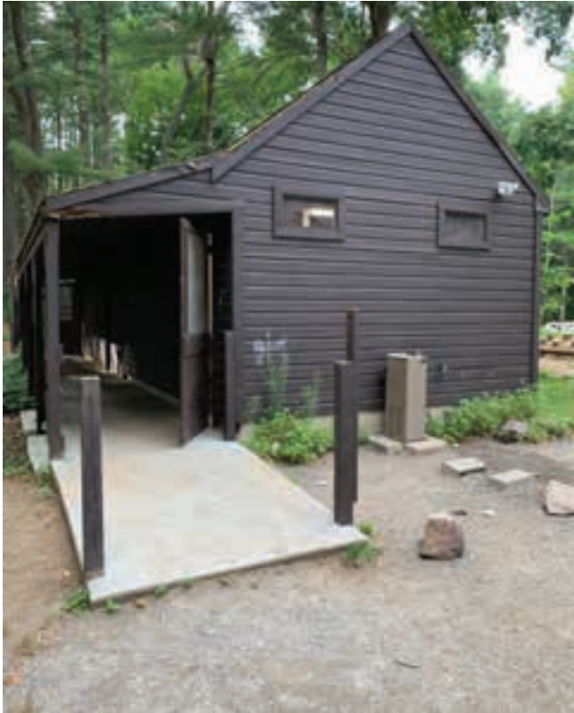
Figure 2-84. The existing stepped ramp and drinking fountain station both show existing accessibility deficiencies.
