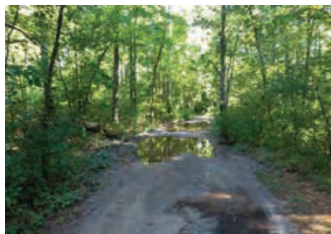
Figure 2-77. Water ponding in some section of the access road and the parking lot
