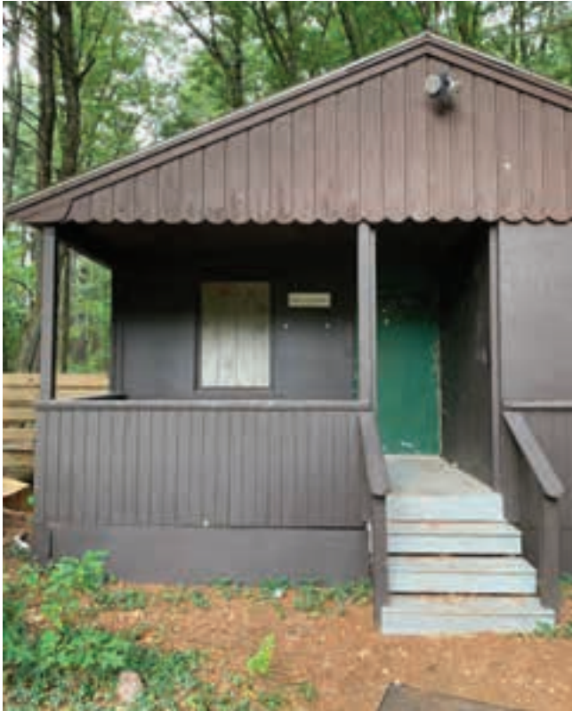
Figure 2-89. The existing Arts and Crafts Cabin. Boarded windows suggest recent inactivity.
