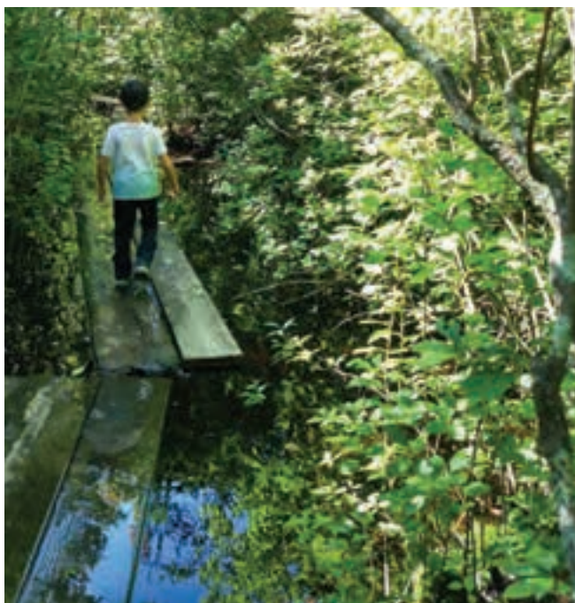
Figure 3-10. Existing unstable and submerged boardwalk at Ponkapoag Bog
