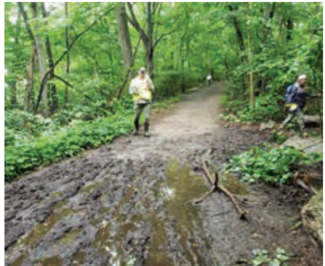
Figure 2-18. Green Dot Trail with drainage problems
