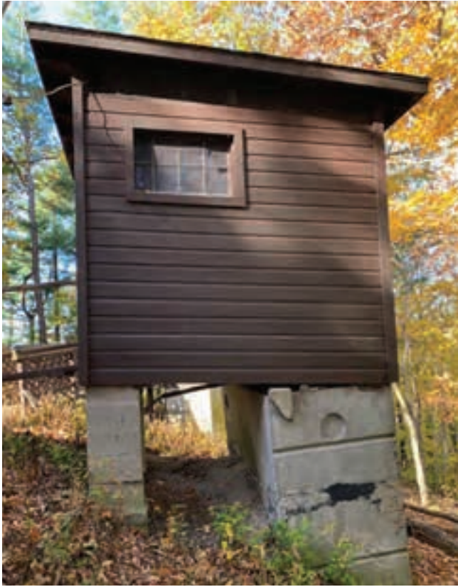
Figure 2-43. Uneven settlement of structural elements
