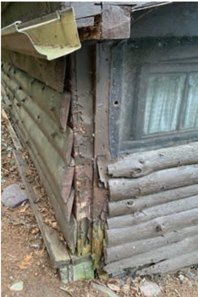
Figure 2-49. Folsom's signs of material degradation due to moisture and insect infestation.
