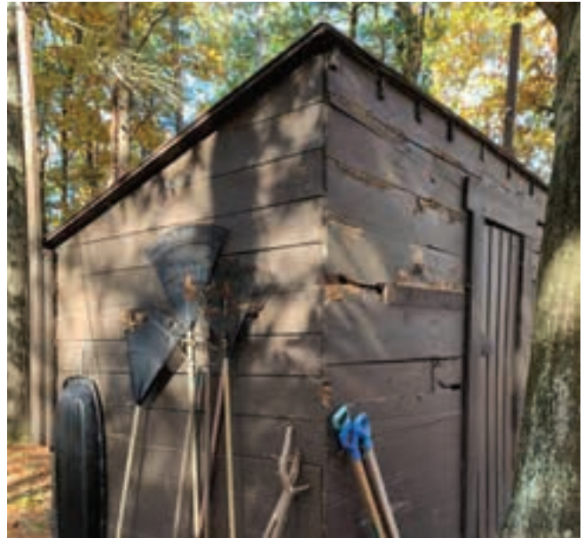
Figure 2-71. Signs of exterior deterioration
