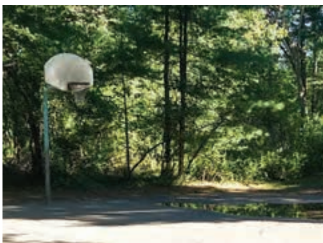
Figure 2-76. Basketball court surface in need of renovation
