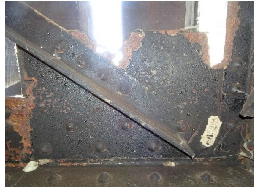
Steel deterioration identified during inspection
