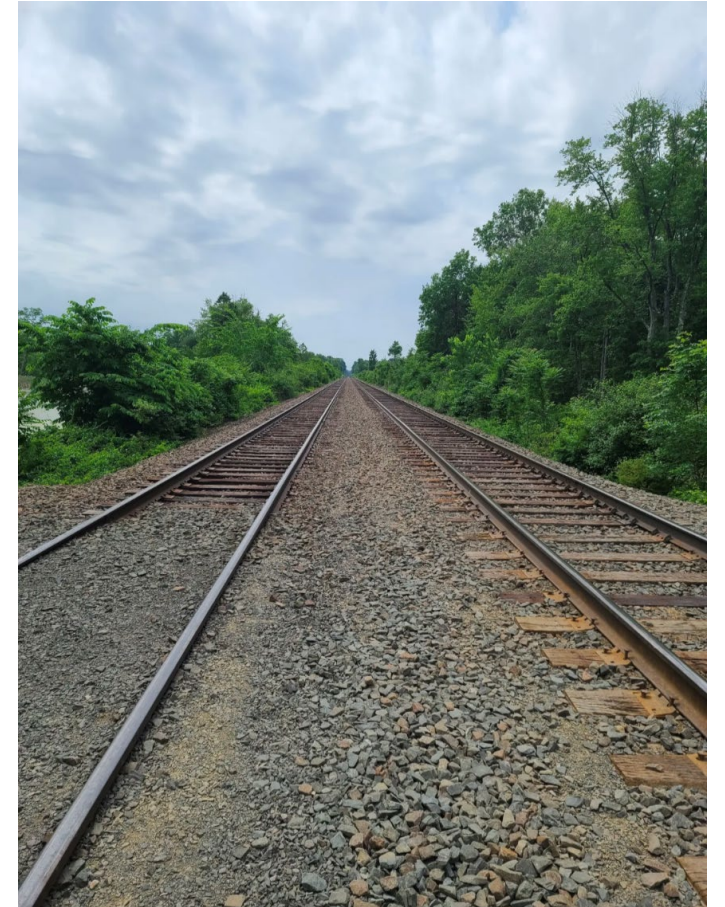
Amtrak's Springfield Line viewed from passive crossing within Fannie Stebbins Memorial Wildlife Refuge in Longmeadow
