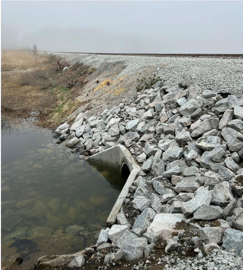
The Cape Main culvert at milepost 63.22 in Sandwich was fully replaced and the far embankment was armored, protecting against future storm surges.
