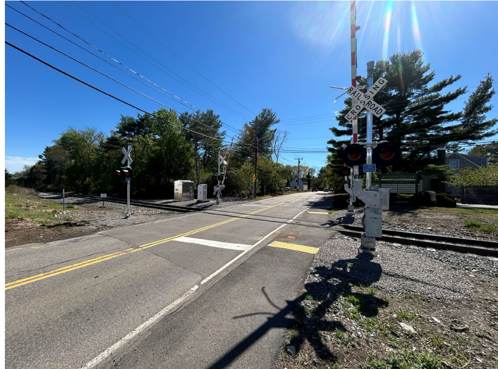
A completed grade crossing upgrade at Elm St. in Foxboro is a part of a series of safety upgrades being constructed along the Framingham Secondary rail line.
