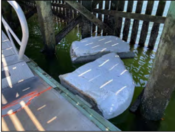
Displaced polystyrene float units after seasonal storm
