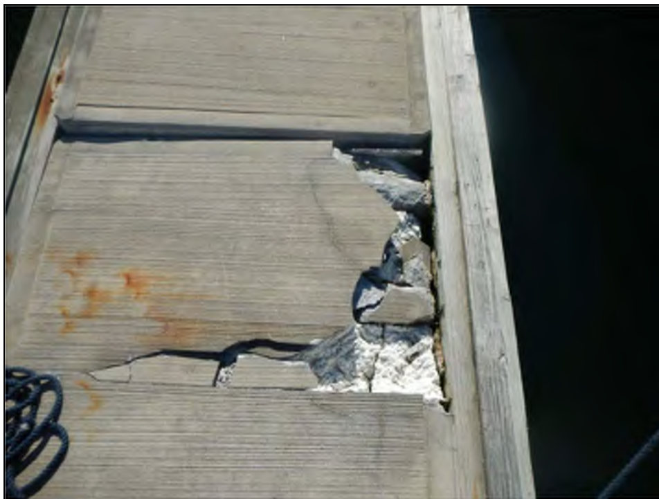
Photo No. 11: Concrete deck deterioration.
