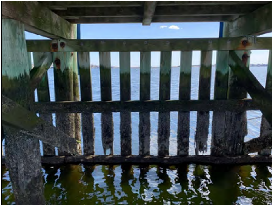
Photo No. 45: Deteriorated timber wave fence.
