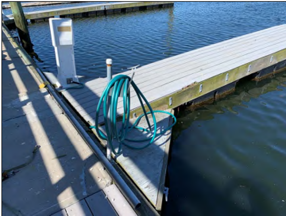
Photo No. 24: Failing timber triangle connection.
