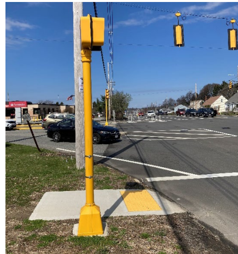
Figure 9. Pedestrian ramp and push button lack connectivity
