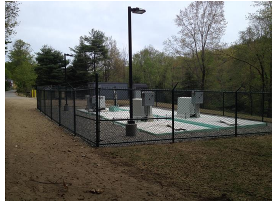
Photo 1.3: Royalston Wastewater Treatment Facility.
