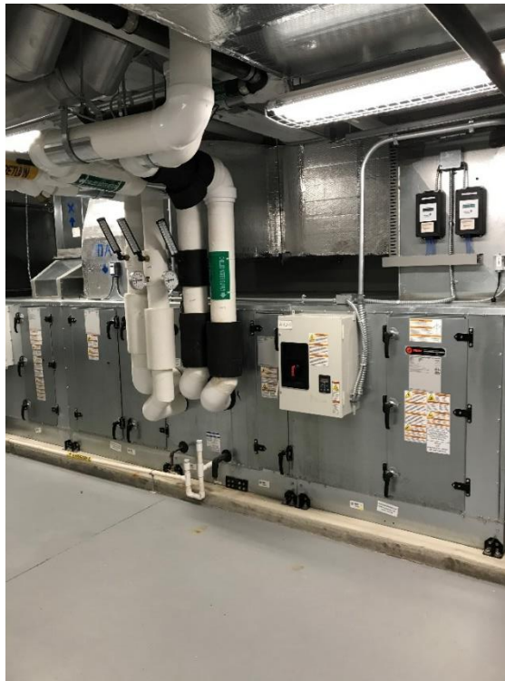
Photo 1 – Representative Air Handler
