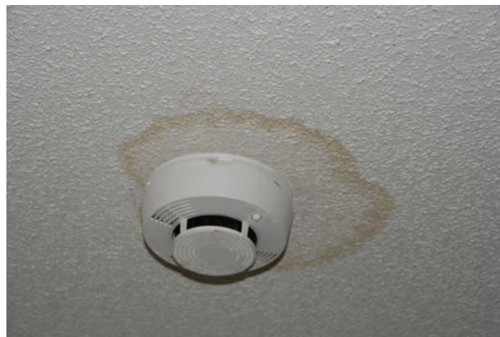
705-1 Development, #21 South Pleasant Street, Apt. 6 – Water Damage Near Smoke Detector
