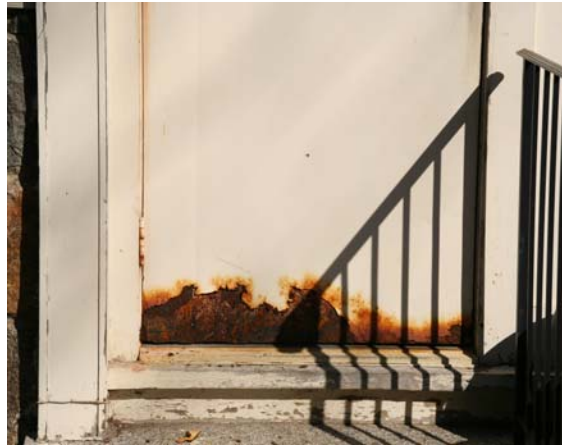
705-1 Development – Outside Door Rusted
