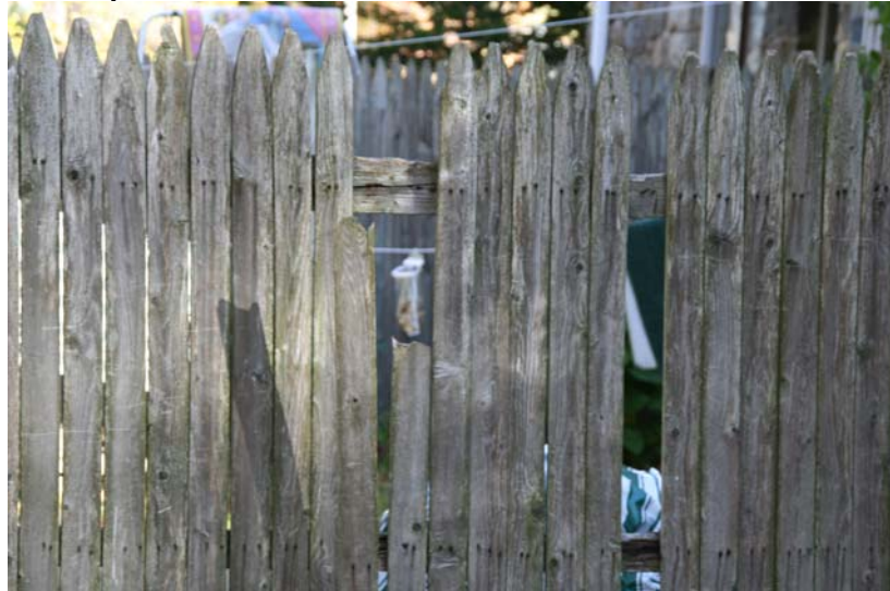
705-1 Development, #21 South Pleasant Street – Broken Fence
