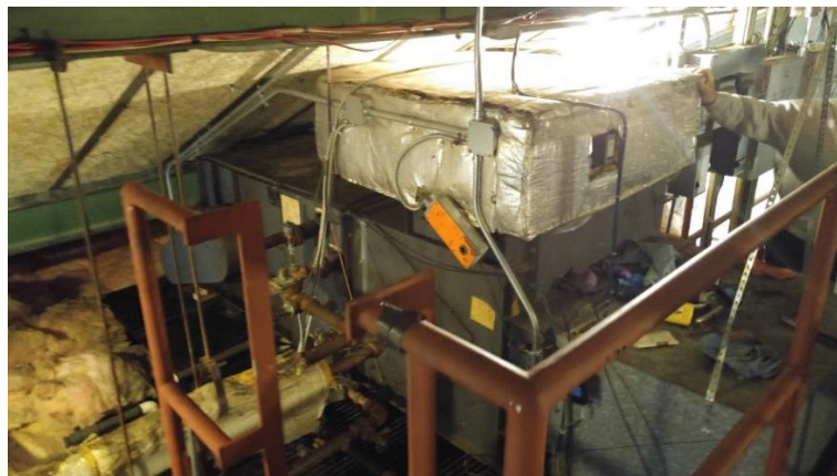
Photo 3: Representative Air Handler (AHU's 3 & 4).
