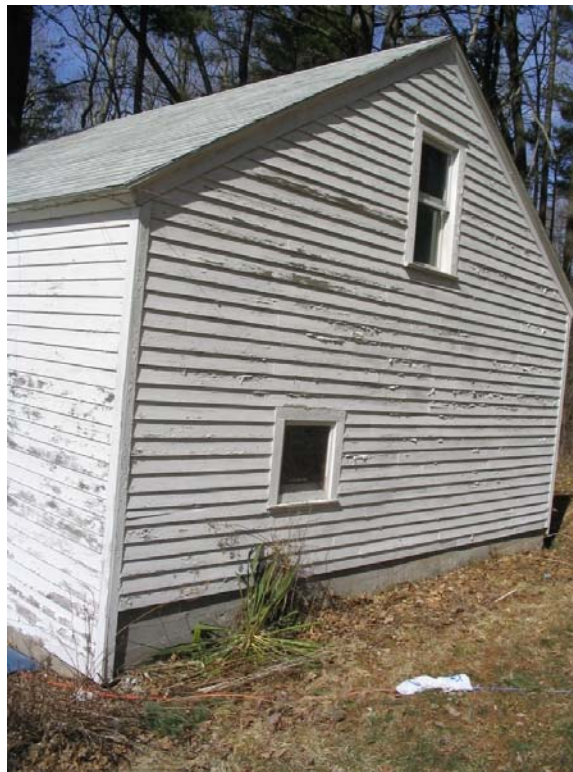
705-2C Family Development, 16 Congamond Road Detached Garage – Peeling Paint
