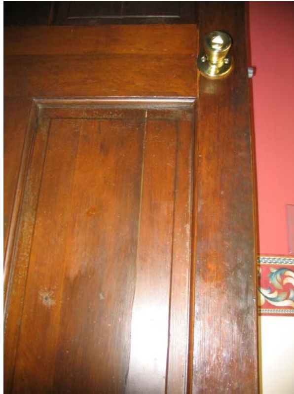
705-2C Family Development, 16 Congamond Road Front Entrance – Door Panel is Cracked
