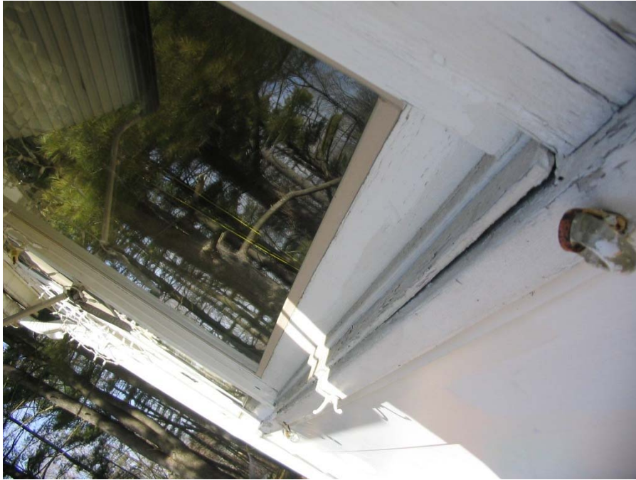
705-2C Family Development, 16 Congamond Road Building Exterior – Wooden Window Sill is Rotting and Peeling
