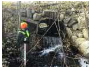
Outlet, Richardson Corner Rd
