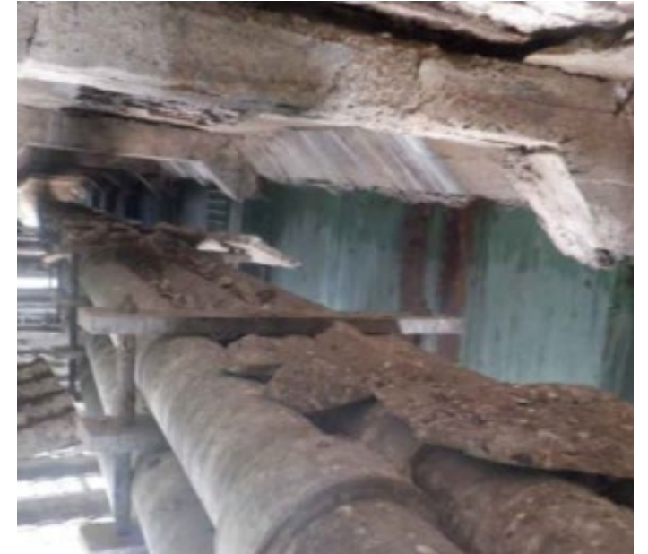
delaminated concrete resting on utility conduits
