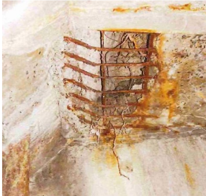
exposed reinforcement bars in bridge structure
