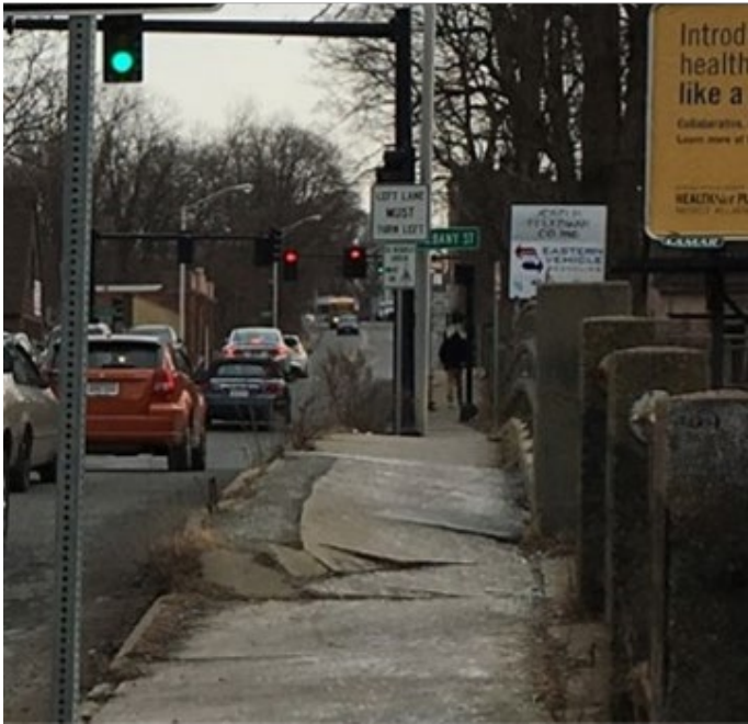
Poor sidewalk condition due to deterioration and heaving
