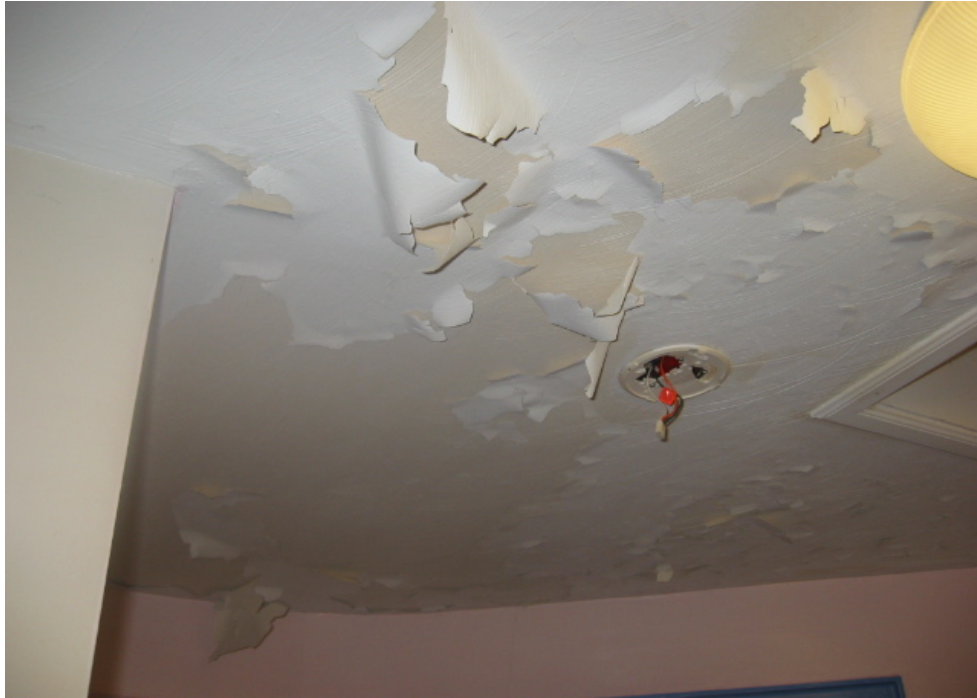
200-C Development, 21 Calthea Street Hallway – Peeling Paint on Ceiling
