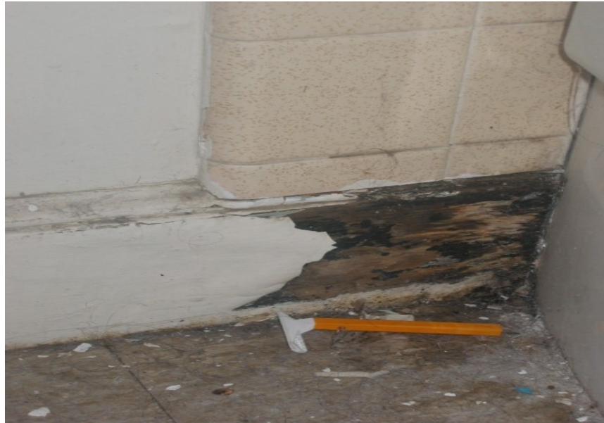
200-C Development, 26 Washington Avenue Bathroom – Floor Board Rotting
