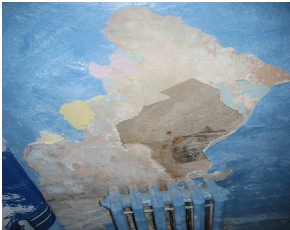
200-C Development, 34 Washington Avenue Bathroom – Plaster Coming Off Wall
