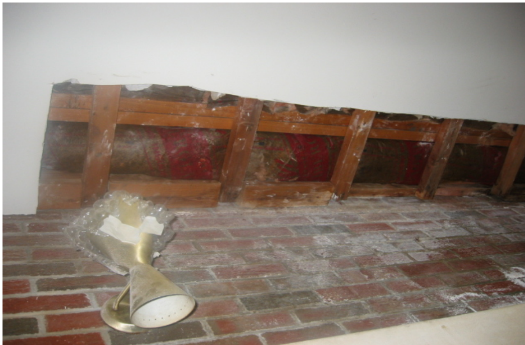
667-C Development, 11 Parker Chase Road Board Room – Hole in Ceiling
