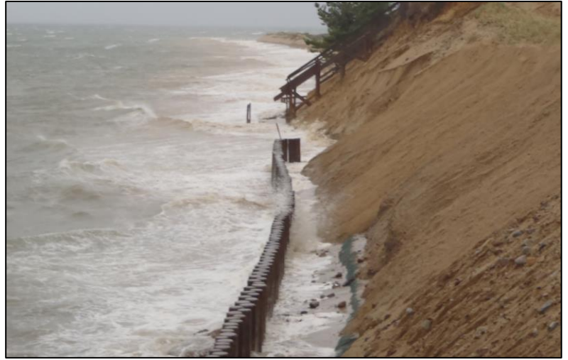
The row of posts installed at the base of this bank is acting like a solid wall, reflecting wave energy and exacerbating beach erosion and erosion of neighboring properties. (Photo: Greg Berman, Woods Hole Oceanographic Institution Sea Grant Program)
