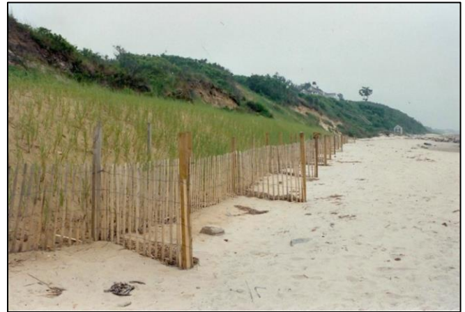
In this project, an artificial dune was built at the base of an eroding bank and heavily planted with erosion-control vegetation. Sand fencing was installed to help trap sand to build the artificial dune. (Photo: CZM)
