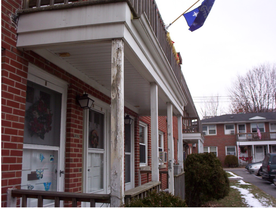
667-1 Development, Duncan Terrace, Building E Peeling Paint on Post
