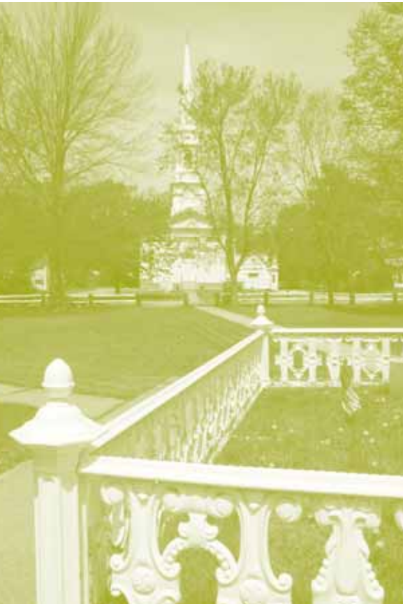
This cast iron fence surrounding a monument on the Barre Commons is in good condition due to regular maintenance.
