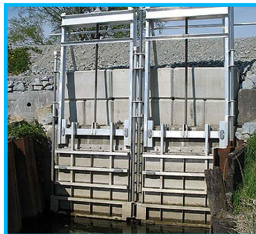
Sluice Gate (actuator not pictured)
