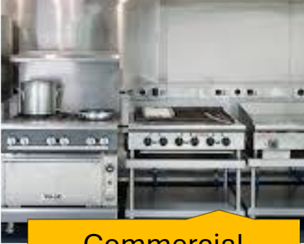
Commercial Kitchen Equipment
