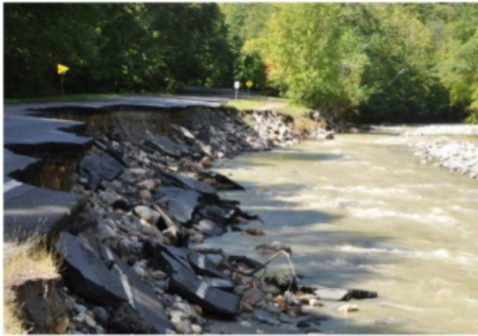
Rt. 2 Hurricane Irene Damage
