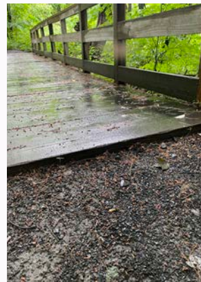
Eroded surfacing creating a change in level or creating an obstacle
