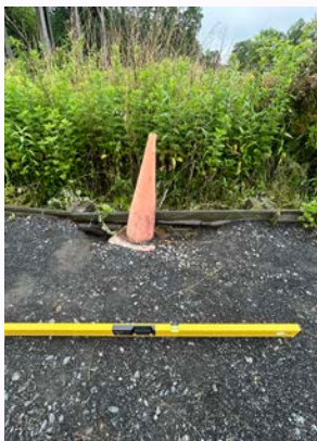
Eroded surfacing caused by drainage
