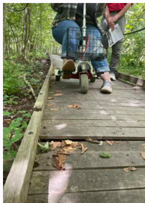
Sunken boards and rotting curbs
