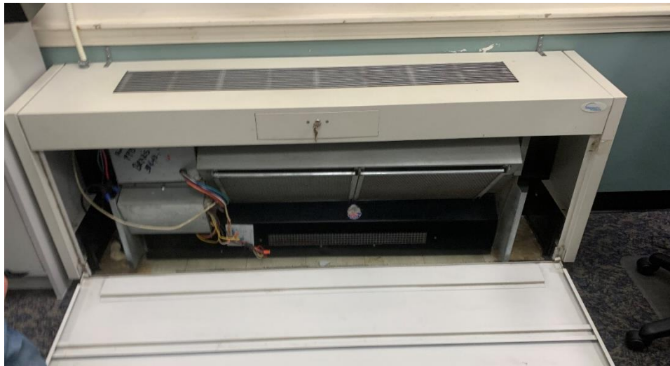
Photo 2 – Typical PTAC unit
