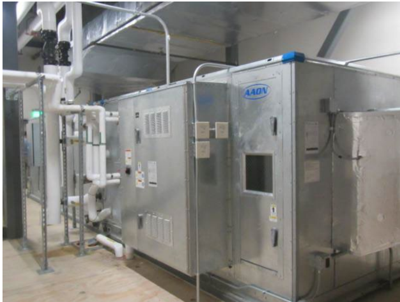
Air handling unit in a mechanical area above the second floor
