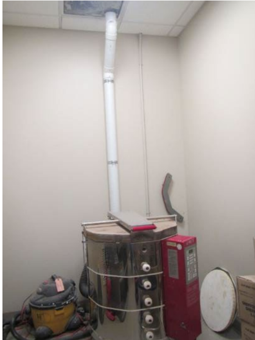
Dedicated kiln vent
