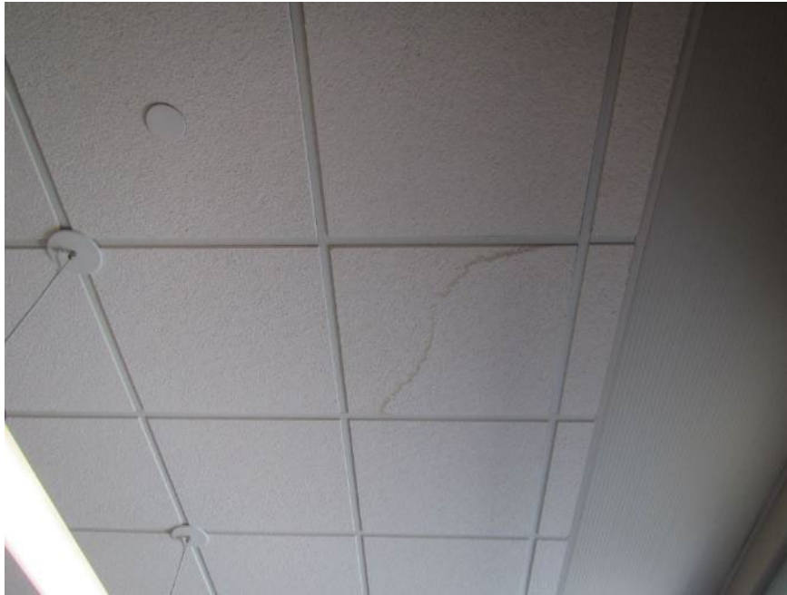
Water-damaged ceiling tile
