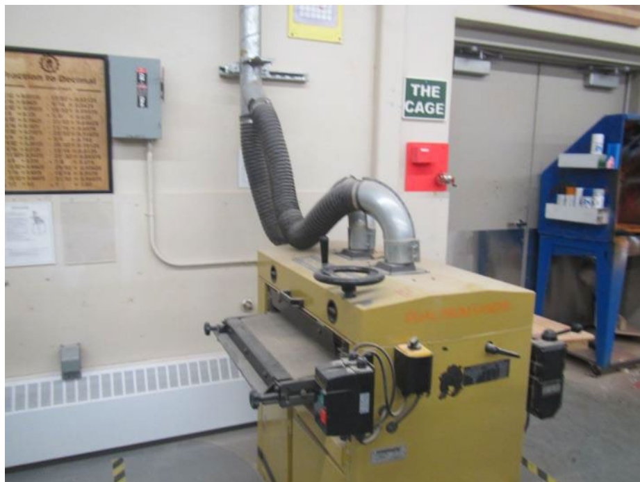
Example of a dust extractor in the wood shop
