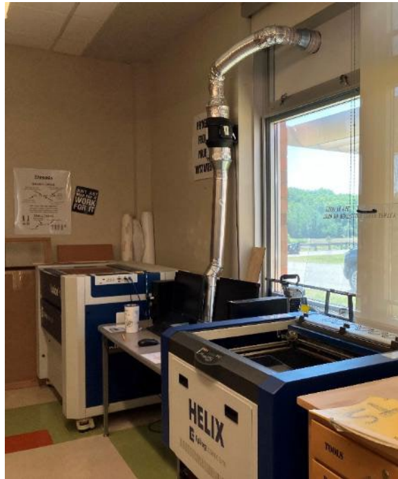
Exhaust vent for a laser cutter
