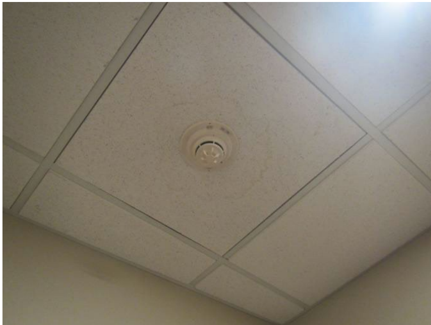
Water-damaged ceiling tile
