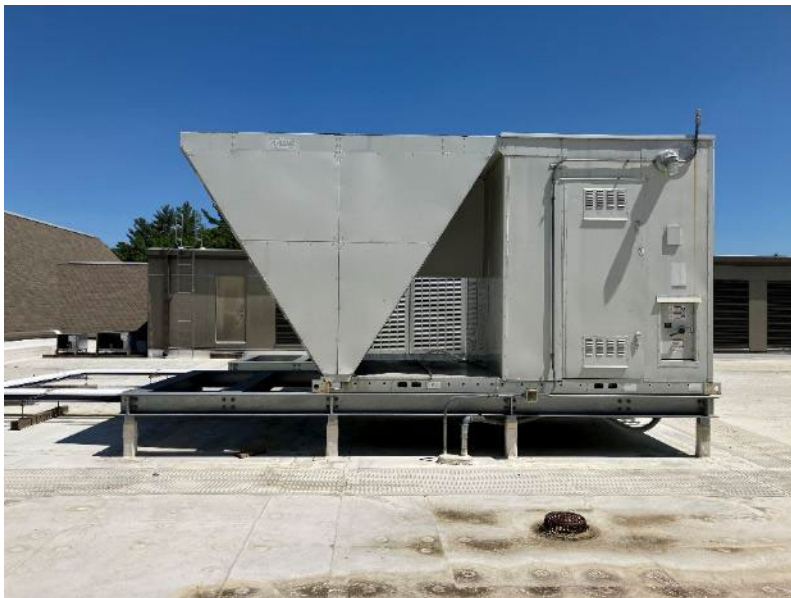
Air handling unit on a flat part of the roof
