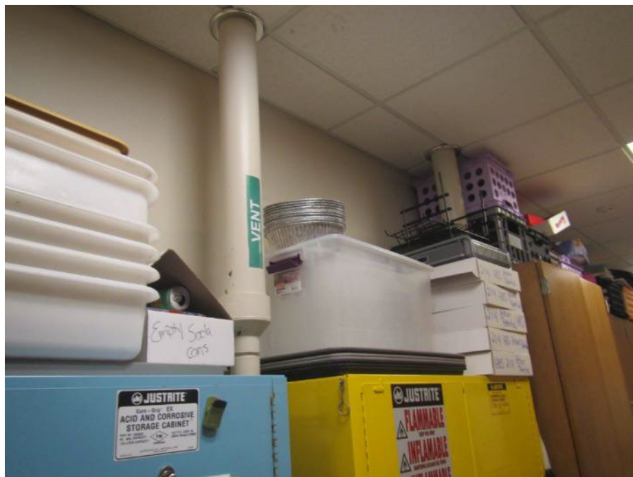
Flammable and acid cabinets with vents
