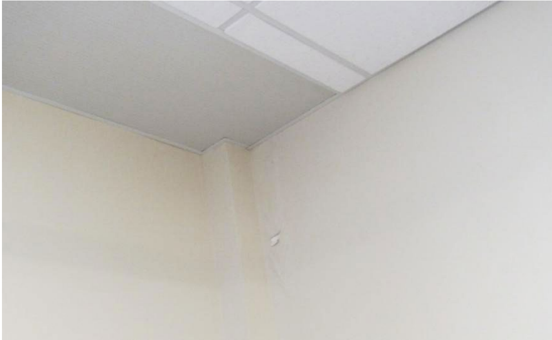
Peeling paint that appears to be due to water damage
