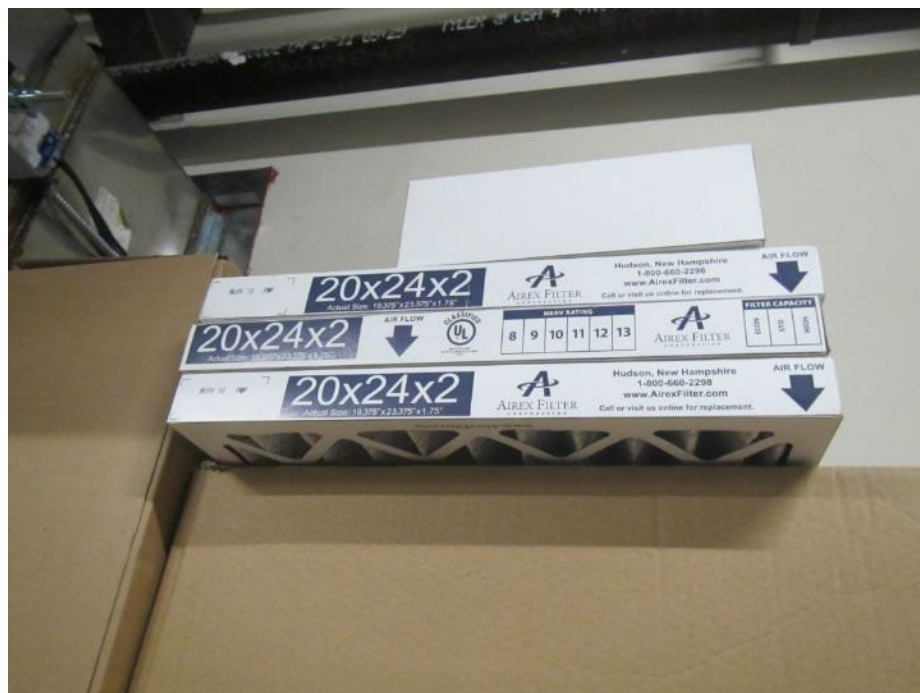
Replacement MERV 10 air filters in an AHU room; filters should be stored in an enclosed space
