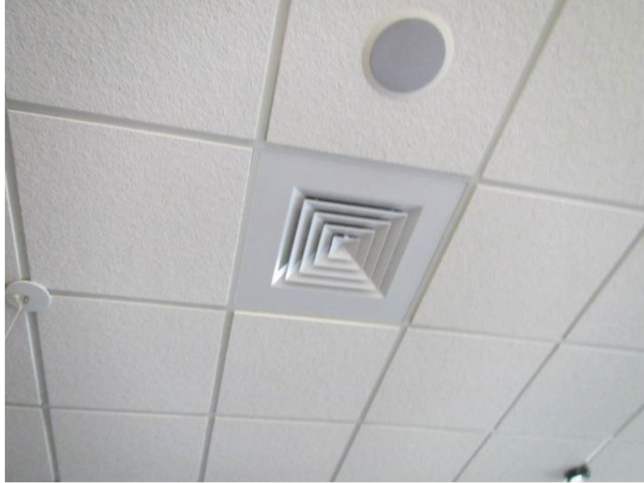
Typical supply vent in a classroom
