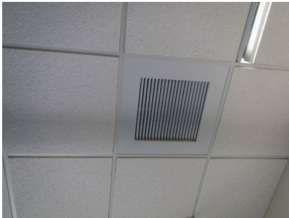
Typical ceiling-mounted exhaust or return vent
