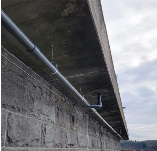
Piping from Cosgrove deck
