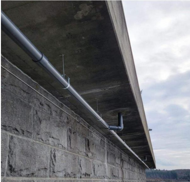
Piping from Cosgrove deck
