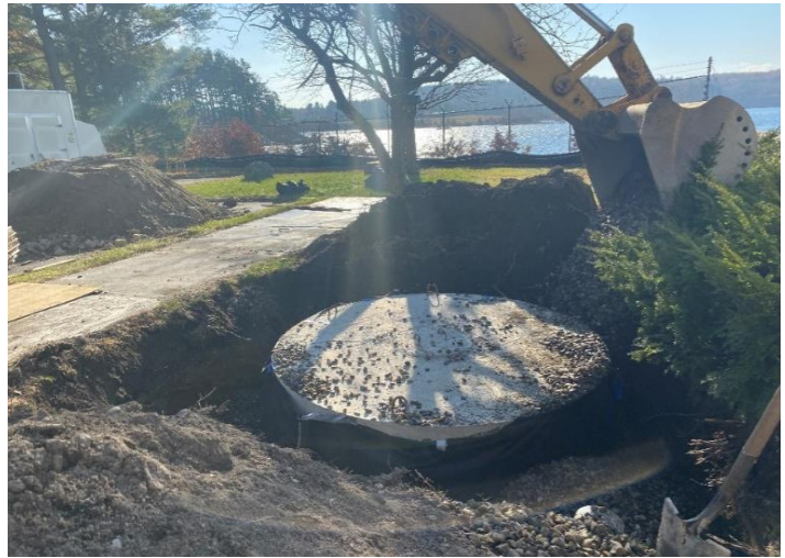
Drywell containing flow from deck drains
