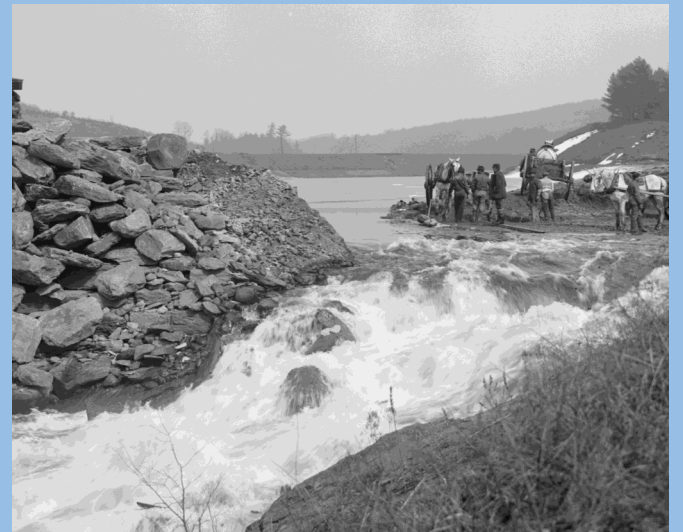
(Above) March 12, 1902. Removing Oakdale Mill Pond dam. Considerable work was done tearing down and cleaning up around the mills.
