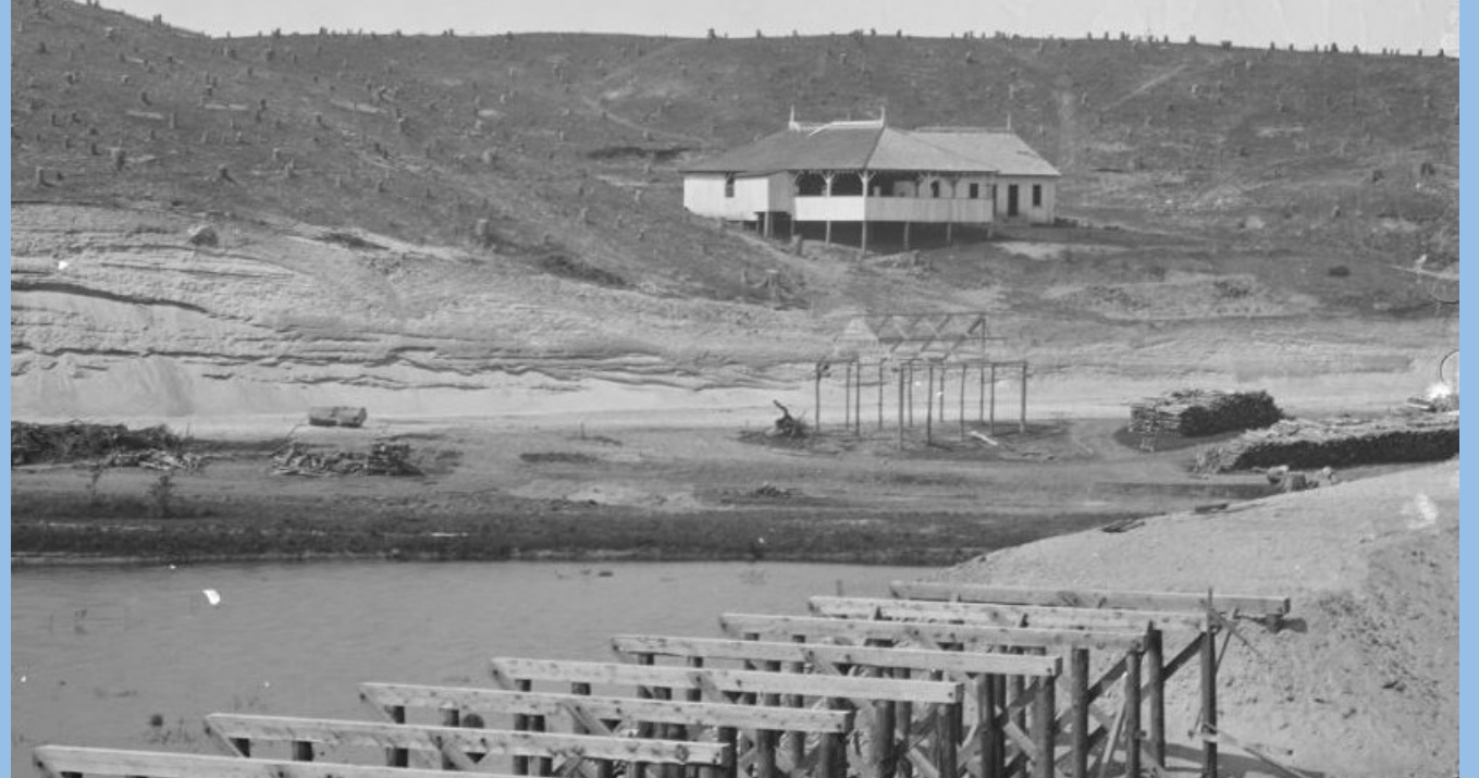
May 1899. Soil stripping at the site of Cunningham's Pavilion, Boylston. All structures and trees were removed before the valley was flooded. Cunningham Ledge is now an island.
