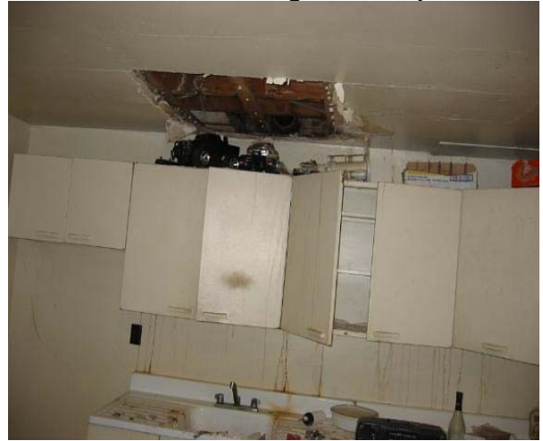
200-3 Development, 17 Gardner Street Kitchen Ceiling Needs Repair
