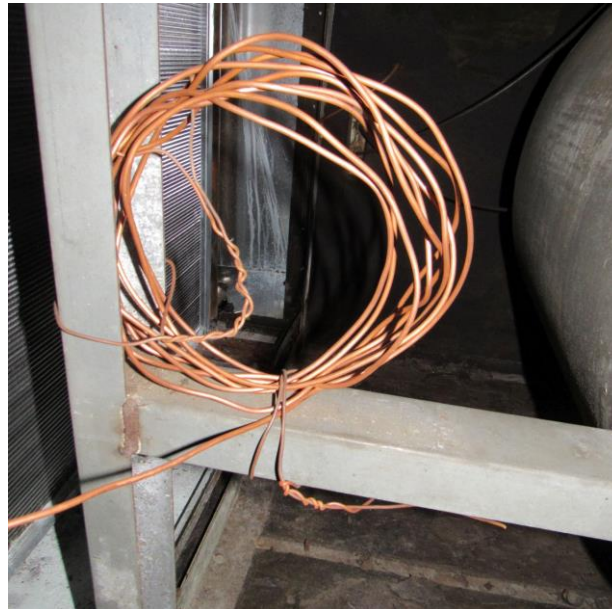
Photo 4 – Improperly Installed Freeze Stat Element
