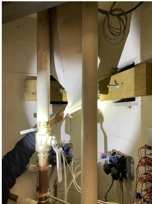
Photo 2 – Capped Exhaust Duct Serving Holding Areas
