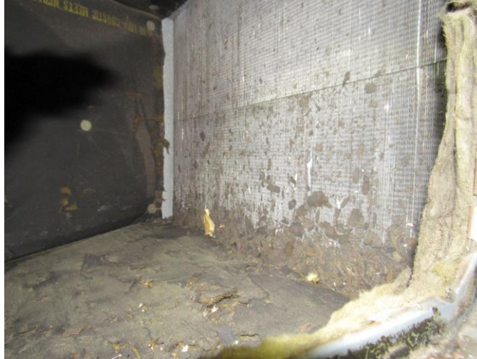
Photo 3 – Deteriorated Duct Liner and Blocked Reheat Coils.
