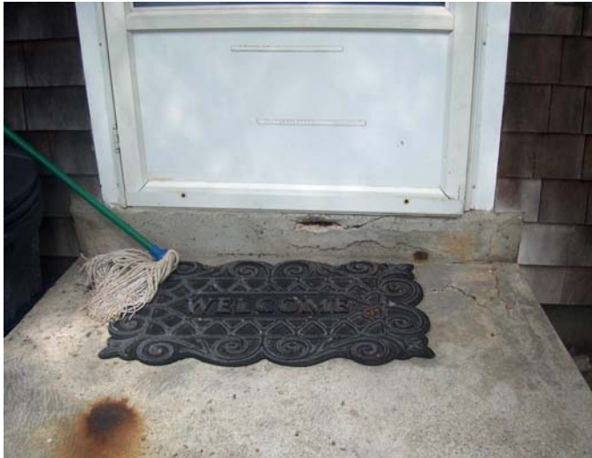
Project 667-1 Entrance Landing in Disrepair
