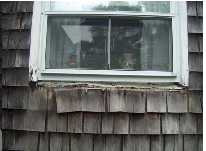
Project 667-1 Window Frame and Shingles Rotting
