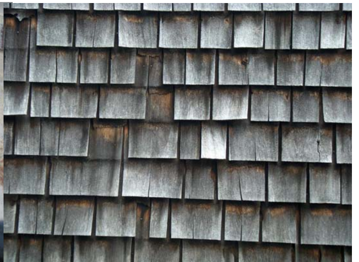
Project 667-1 Missing and Rotting Shingles
