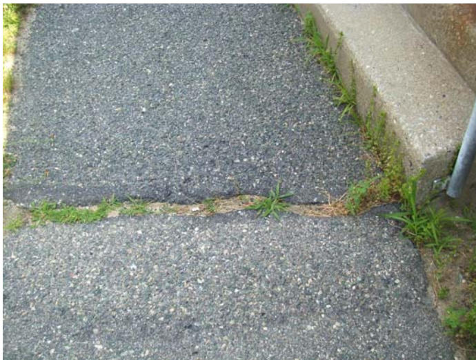
Project 667-1 Crack in Sidewalk
