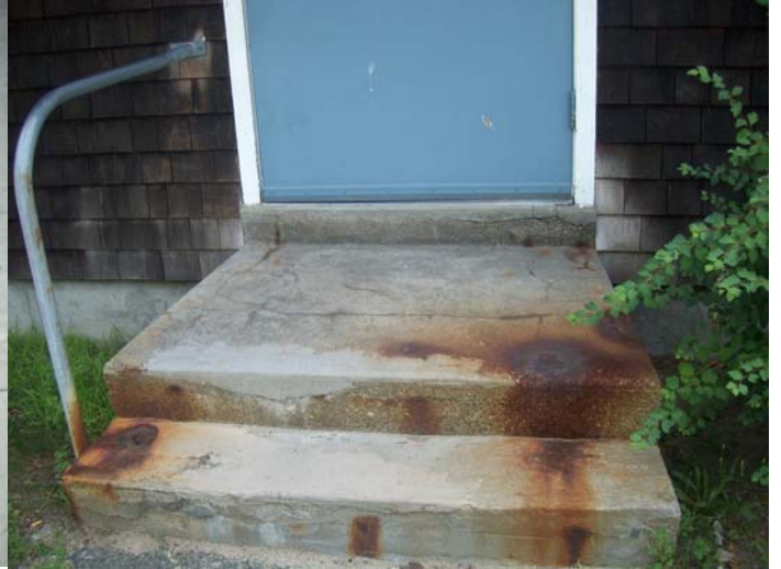
Project 667-1 Community Room Steps Rusted and Cracked
