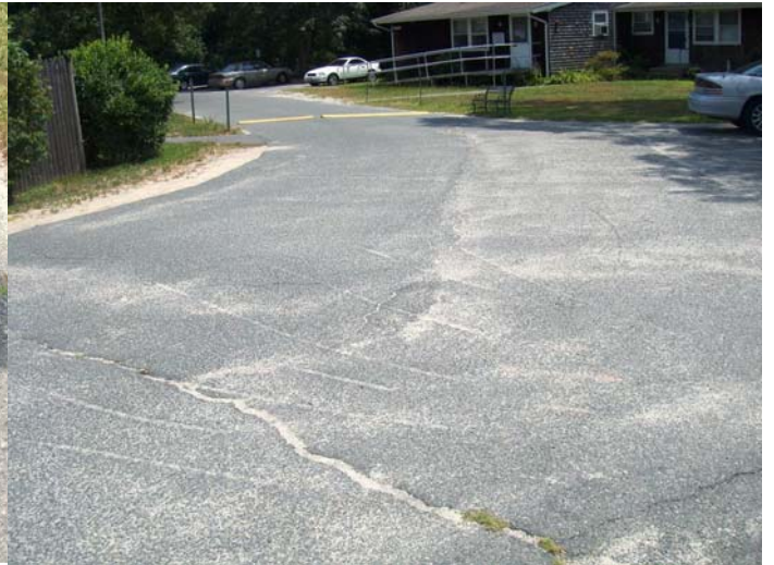
Project 667-1 Roadway Cracked and in Disrepair
