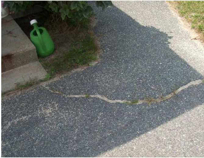
Project 667-1 Walkway Cracked
