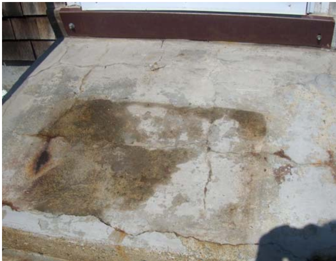
Project 667-1 Front Entrance Landing Cracked
