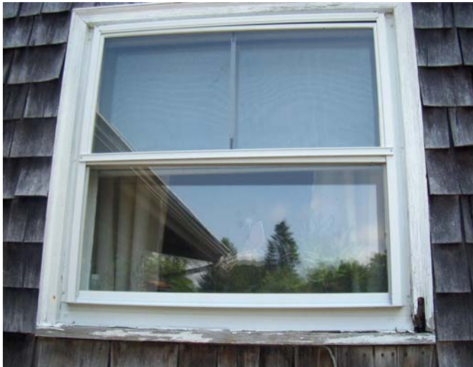
Project 667-1 Window Frame Rotting
