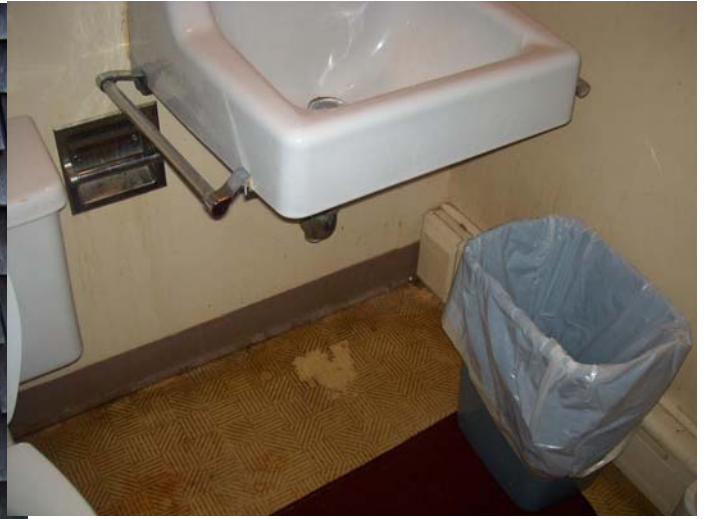
Project 667-1 Bathroom Floor in Disrepair
