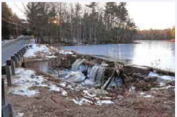
Historic dams in Massachusetts were not designed to handle the increasingly heavy rain events driven by climate change and many have aged past their life span. Wendell has three significant hazard and two low hazard dams that could destroy critical facilities and infrastructure, and impact residents, property, and the environment if they failed. Bowens Pond is pictured above. Photo by Greenfield Recorder.
