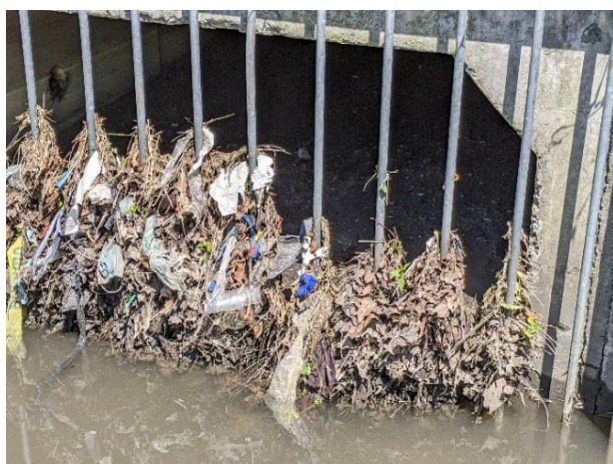
Photo C-7: The box culvert outlet had a grate clogged with organic debris and trash. Behind the grate, the sediment buildup can be estimated at 1 foot deep.
