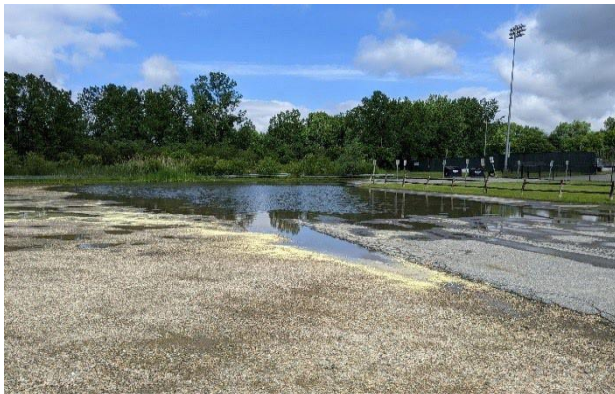
Photo C-1: Looking toward the West where the constant flooding in the parking lot is a major concern.
