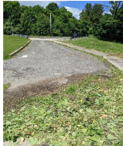
Photo C-6 (right): The end of the road near 17 Francis Ave showed signs of high sediment deposition, vegetation, and a clogged catch basin (not found).
