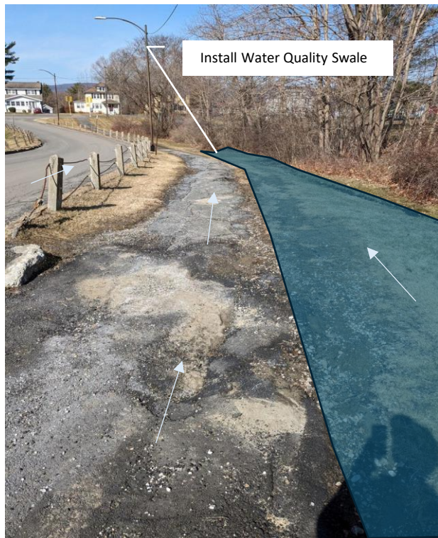
Photo C-21: Existing ditch and crumbling pedestrian accessway.
