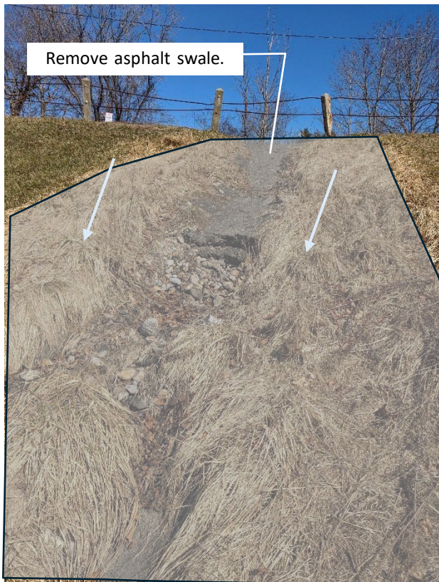
Photo C-25: Erosion at the asphalt swale along the south side of the entrance road to the school.
