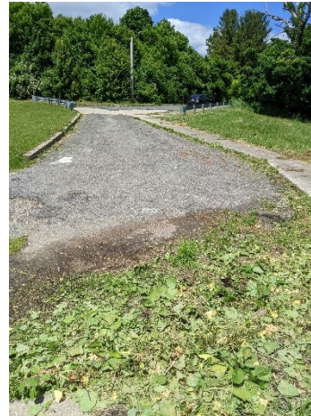
Figure 2: The end of the road near 17 Francis Ave showed signs of high sediment deposition, vegetation, and a clogged catch basin (not found).
