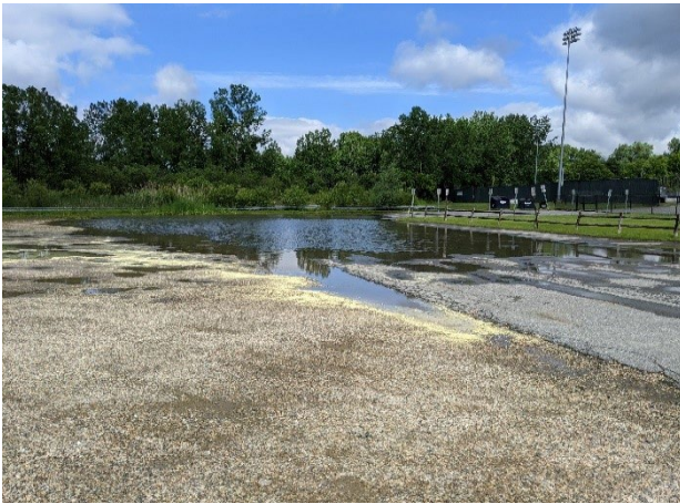
Figure 1: Looking toward the West where the constant flooding in the parking lot is a major concern.
