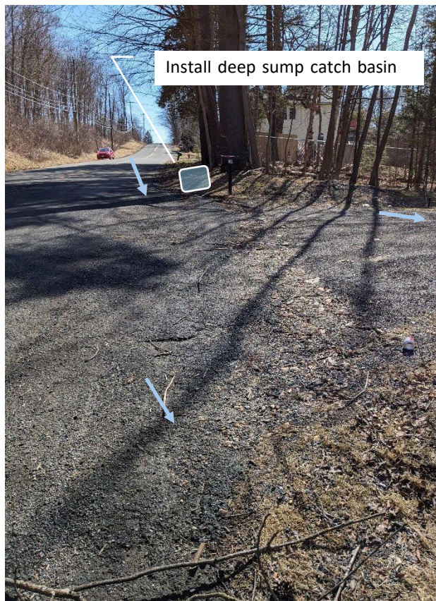
Photo C-27: Erosion at the intersection of Spring Street and Bull Hill Road.
