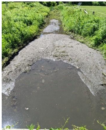
Photo C-8: The sediment deposit at the outlet of the box culvert. Some larger riprap can be seen in the plunge pool while the mounding and rest of the swale are filled with fine sands and finer sediment.
