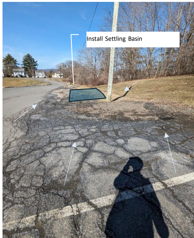
Photo C-22: Loose sediment and erosion occurring at the edge of the parking lot
