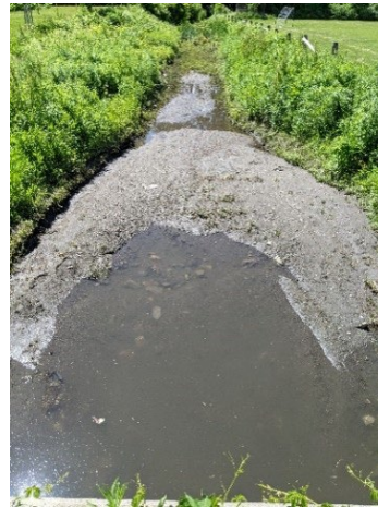
Figure 2: The sediment deposit at the outlet of the box culvert. Some larger riprap can be seen in the plunge pool while the mounding and rest of the swale are filled with fine sands and finer sediment.
