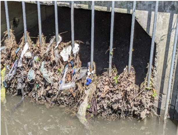
Figure 1: The box culvert outlet had a grate clogged with organic debris and trash. Behind the grate, the sediment buildup can be estimated at 1 foot deep.
