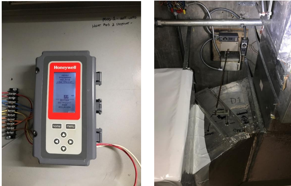
Photos 4 and 5 – Programmable Controller and Outdoor Air Damper Controls for AHU-2
