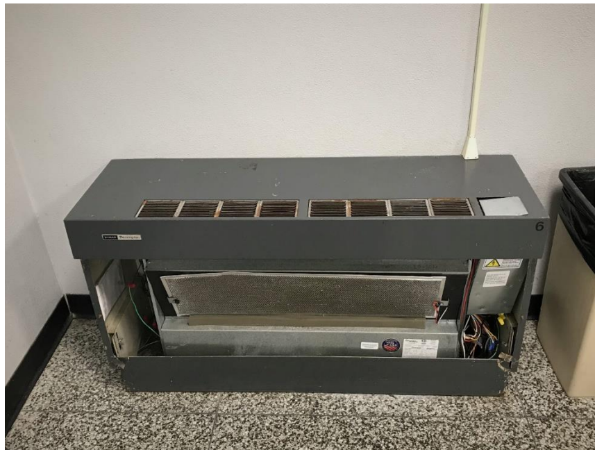
Photo 2 – Original Unit Ventilator
