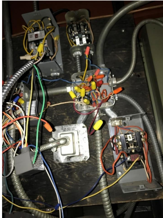
Photo 3 – Original Controls for AHU-1
